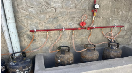
Gas Line maniFold
