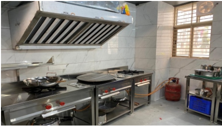
SS Exhaust Hood
